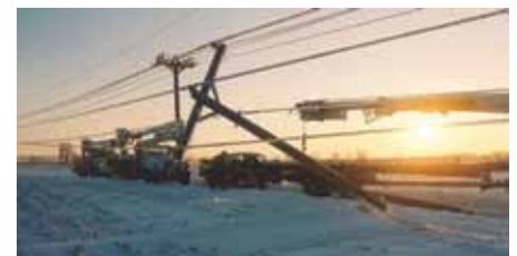
Power outages due to snow and ice storms are especially threatening because of extreme cold temperatures.
